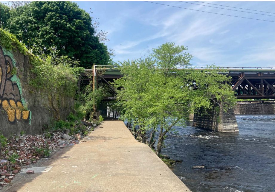
Looking west along the Merrimack River Rail trail towards the former rail bridge that will carry the Lawrence Manchester Rail Trail
